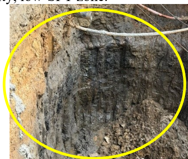
Figure 8. The condition of the soil is saturated with water, according to geoelectric results there are pockets of water at that depth.
